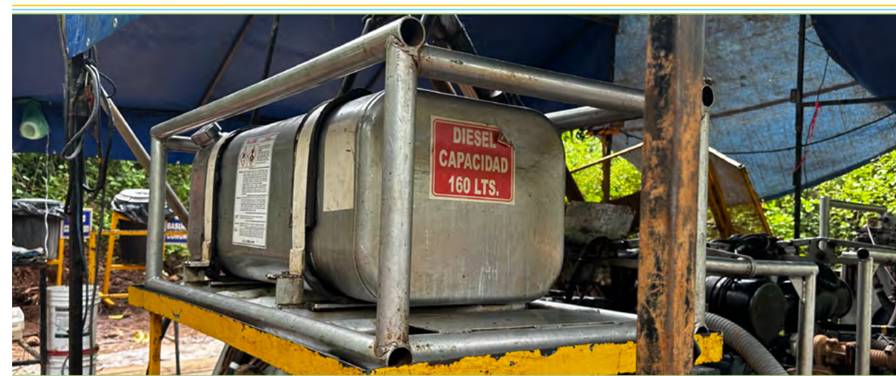
Environmental surveillance on drilling areas: fuel container - hazardous substances management
